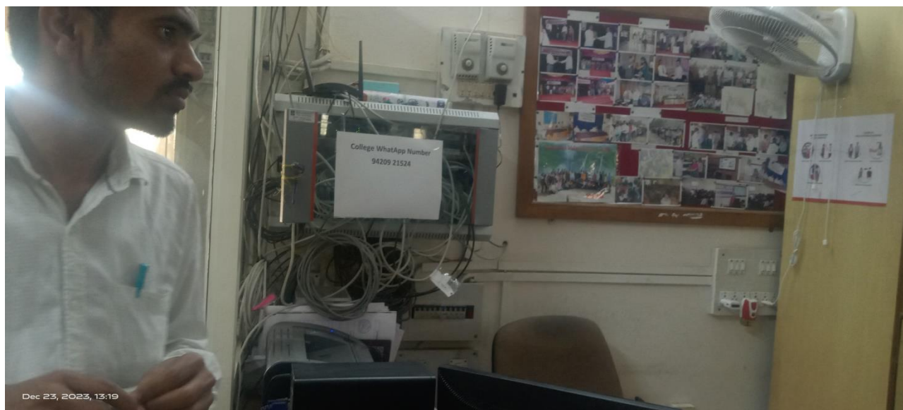
Plate 13: Exposed wiring in the computer laboratory areas
