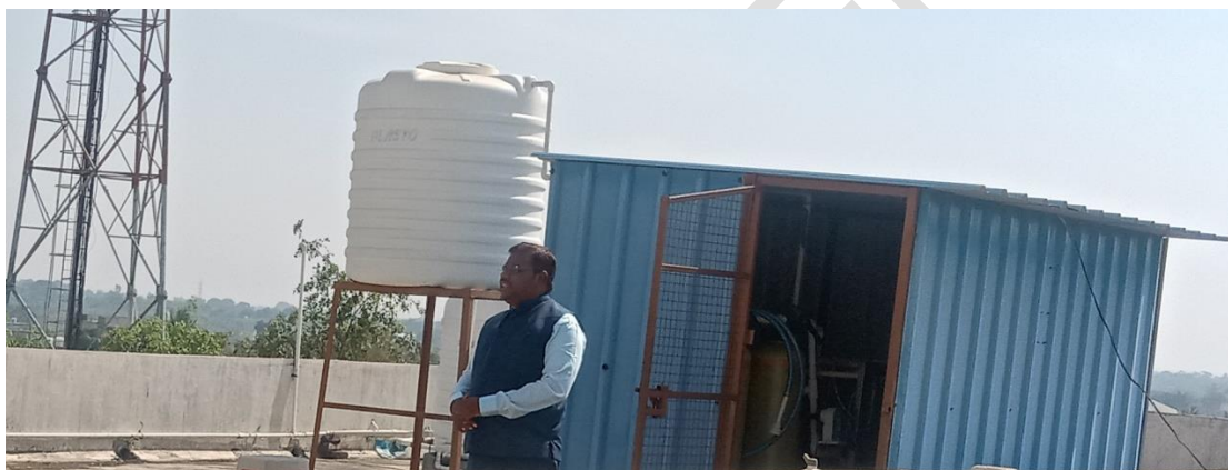
Plate 5: RO facility and overhead water tanks in the premises
